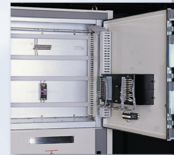
저압실 (Low Voltage Compartment)
